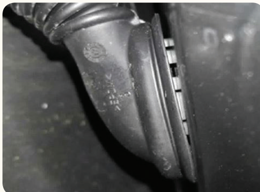
Improperly installed grommet
