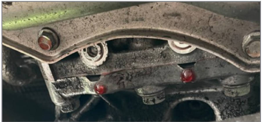
Fluid leaking from the weep holes.
