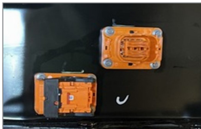
High-voltage battery pack without the rear ground strap bracket.
