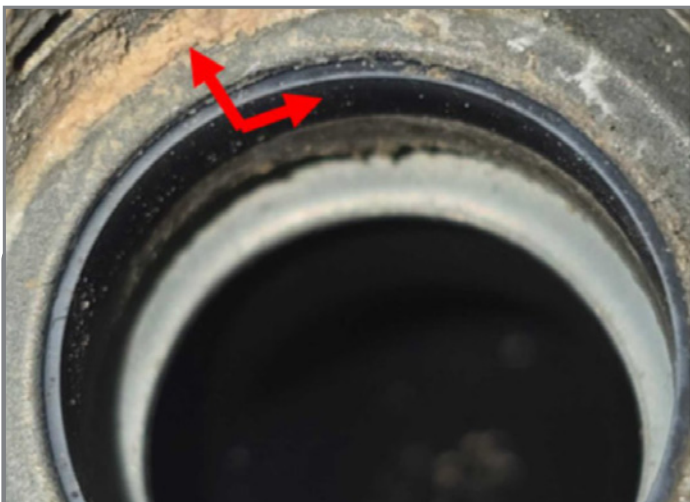
Failed lip seal
